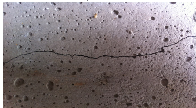
Figure7. Sample with Cracks Due to Manual External Loading
